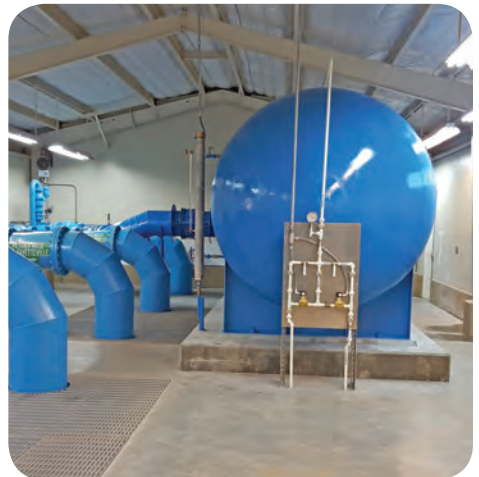
Surge Tank installed and operational.
