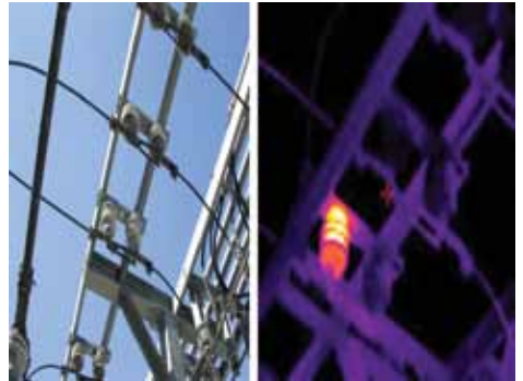
The photo at the left shows what you see with the naked eye. A photo of the same structure, taken with a thermal imaging camera, reveals a hot spot that needs to be addressed.
